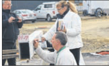
Photos courtesy of Ryan Berry | DarkeCountyMedia.com Employees and community members signed the steel beam before it was put into place.
